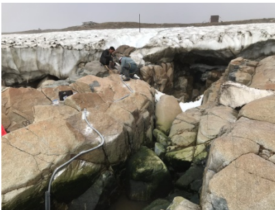
Figure 8. Picture of a vented pressure tide gauge installed for tidal datum determination on St. Lawrence Island, Alaska. Field crew is securing air hose that runs from below MLLW to the electronics enclosure on top of the hill in the background.
